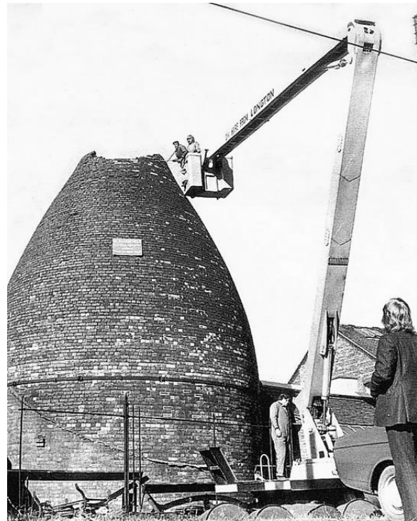
Fig.4.4 Hovel oven manual demolition, working from the top courses down using cherry picker crane access for safety c1969.
