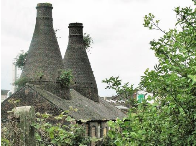
Fig.4.7 Abandoned twin bottle ovens at the former Falcon Works, Stoke illustrating how vegetation can readily take hold on the upper edges of the inclined brick courses *
