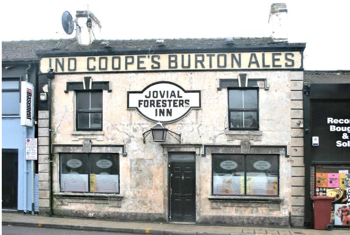
Fig.2.15 Hanley Marsh Street, Jovial Foresters Inn. Decline can often follow the lack of maintenance *
