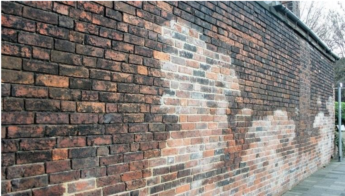
Fig.2.46 Brickwork repairs, Hanley surrounded by surface blackening occasioned by pollution *
