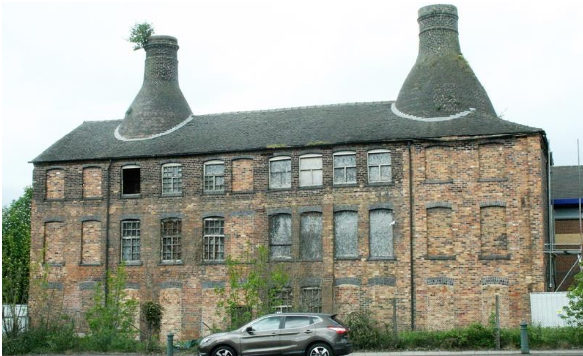
Fig.2.38 Bottle oven stacks penetrating and contained within the former Tams Factory, Commerce Street, Longton *
