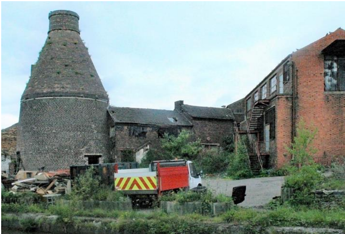
Fig.8.24 Grade 2 Listed bottle ovens and adjacent factory buildings, Longport needing care and attention *
