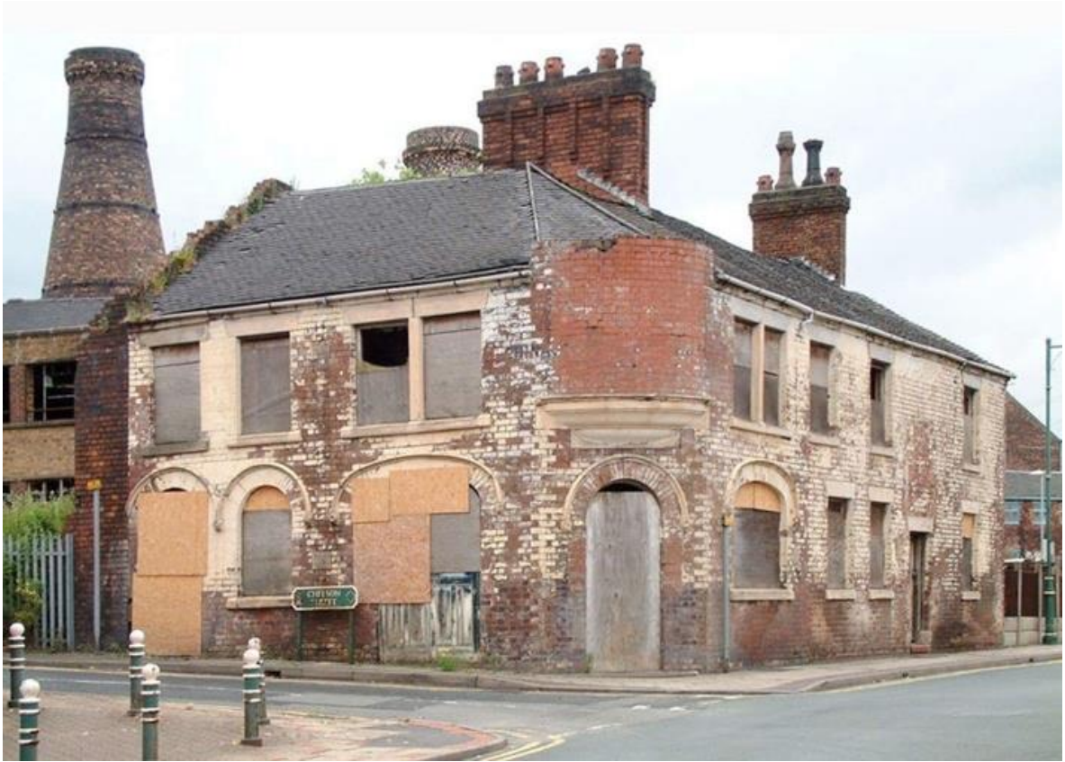
Fig.9.4 A CoRE scheme before repair and restoration work, Normacot. Image: Anthony Williams
