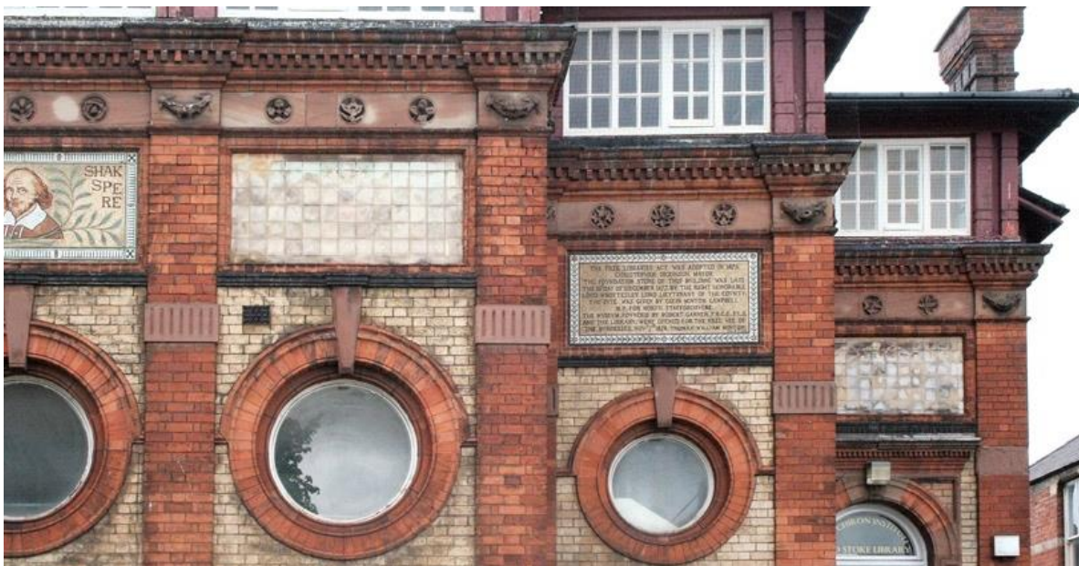
Fig. 9.1 Stoke-Upon-Trent Library decorative brickwork and tiles depicted local scenes, although the tiling is now extremely faded *
