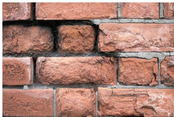
Fig.2.44 Eroded local soft red brickwork with cinder mortar using fly/flue ash from burning coal; and later cement-based pointing *
